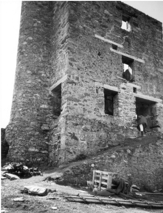
The man-engine house in May 2003 with the author peering into the doorway opening. The pillar of stonework to his left has been rebuilt to fill in the gaping hole left by the scrapmen a century ago. All the lintels have been replaced with Irish oak and selective repointing carried out. Photo. Roz Cundick.
