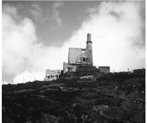
Some scaffolding remains in place on the boiler-house side of the house for possible re-use in stages 2 and 3. Note the temporary props beneath the man-engine loading block, left of the house, where the bolt tunnel lintels have rotted away. These are being replaced. Photo. Roz Cundick.
