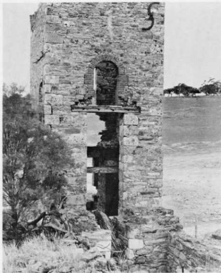
Bull Cornish enginehouses on mining sites are exceedingly rare. The cylinder was suspended over one side of the shaft, with the enginehouse curtailed to prevent total obstruction of the shaft for hoisting pitwork etc. Above: The complete house of a 48-in Bull erected 1861 at North Rhine copper mine, S. Australia in 1861. This rear view shows remains of the timber auxiliary-cum-balance beam, which was beneath the cylinder, lying half in the house. Above right: Front view of Harvey-built 45-in Bull enginehouse at Farler's Pit, Nailsea, Somerset. It worked 1848-61 and the cylinder stood half in and half out of the open-fronted house. The auxiliary beam was overhead.
