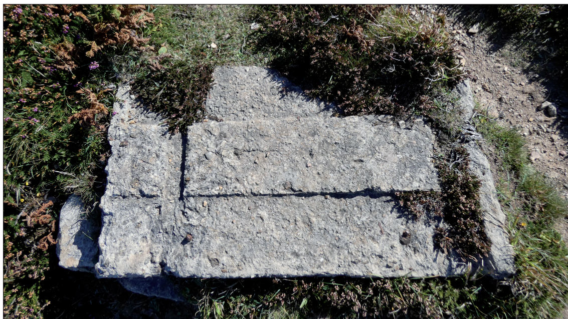
Cut granite support for the tramway, on the north side of the building shown opposite. The tram rails were made from timber throughout, rather than just outside the danger area buildings.
