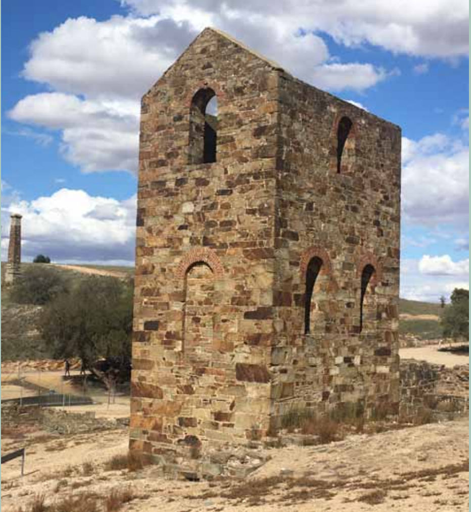
Fig. 14: Rear view (with in-filled cylinder opening) of Morphet's 20-inch winding engine house at Burra Mine.
