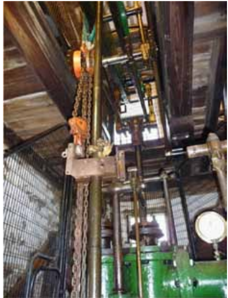
Above: chain block in position for lifting Air pump from Hot well.
