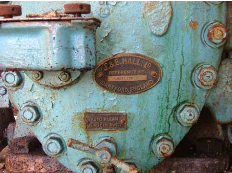
Refrigeration compressor by J & E Hall of Dartford in the old brewery.
